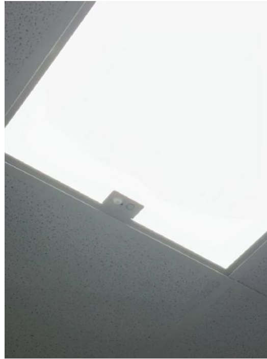
Figure 5: Integrated sensors with wireless control can offer enhanced control capabilities in retrofit situations such as in this 2x2 foot edge light LED panel, which replaced a standard 2x2 foot acrylic lensed fluorescent troffer. Courtesy: McGuire Engineers
