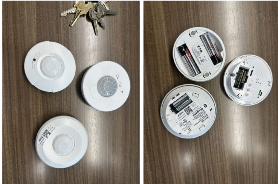
Figure 2a/b: Many wireless sensors are now battery powered which can provide significant flexibility in placement. However, batteries do not last forever and future maintenance must be factored into any design. Courtesy: McGuire Engineers
