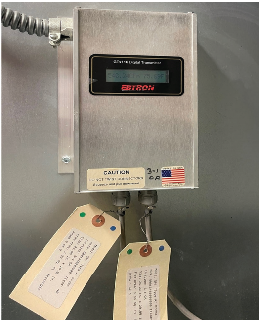
Since its installation in 2009, the airflow measurement station has remained accurate and reliable.
