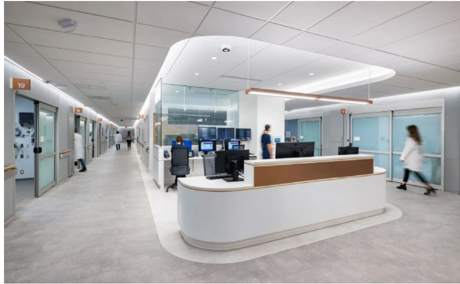
Figure 1: Caregiver station with central touchpad to control corridors. Courtesy: HDR, Dan Schwalm PennFIRST
