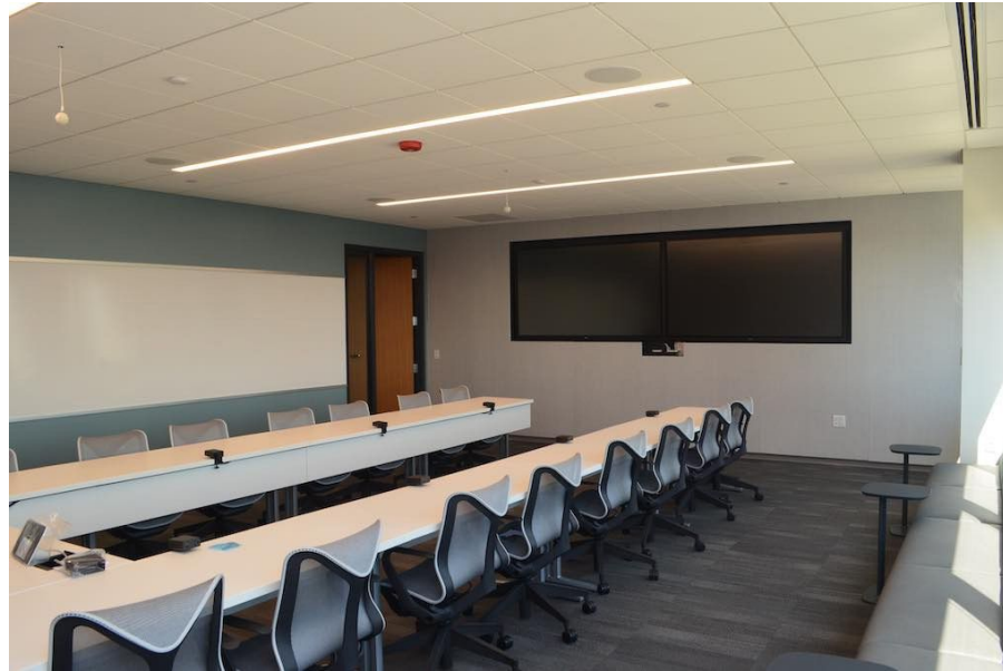
Figure 1: Install example showing wall controls and combination occupancy sensor/photocell. Courtesy: SmithGroup
