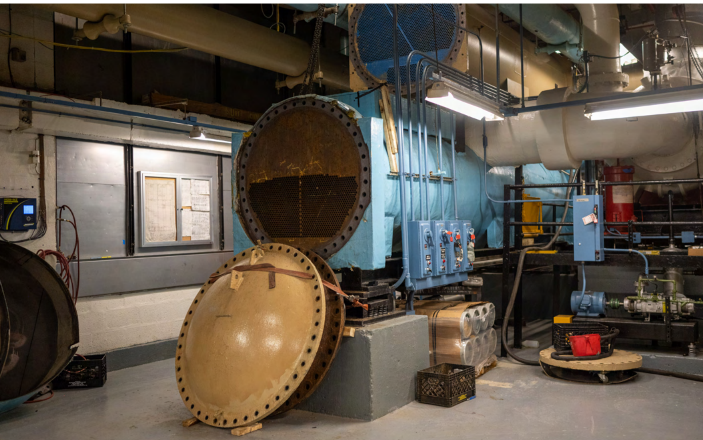
HVAC solutions need maintenance to maximize performance and minimize downtime.
