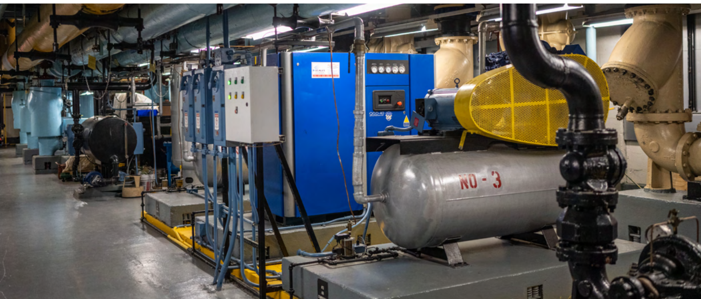
Even the cleanest mechanical room is not a hospitable environment for a standard off-the-shelf PC.
