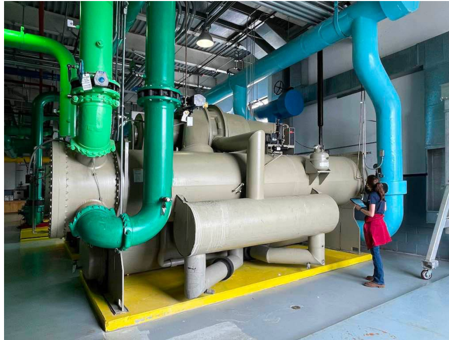
Mechanical HVAC equipment in a major hospital in Dallas Fort Worth. Courtesy: LAN
