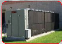
CHILLER COIL INTAKE FILTERS
