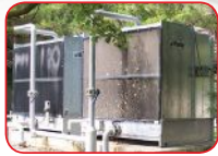
COOLING TOWER INTAKE FILTERS
