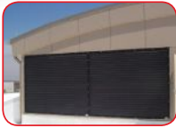
LOUVER INTAKE FILTERS
