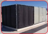
ROOFTOP UNIT INTAKE FILTERS
