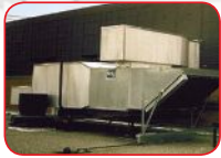
AIR HANDLING UNIT INTAKE FILTERS
