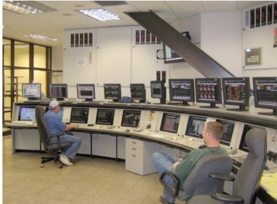
Figure 1: Modern technology allows owners to consolidate controls into a single management center that acts as a gathering point for data produced by essential property systems. Courtesy: Stanley Consultants
