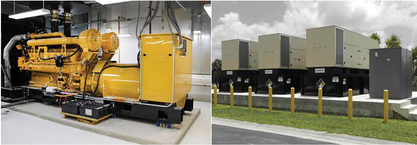
Figure 3: Example of an indoor (left) and outdoor (right) generator installation. Courtesy: WSP USA
