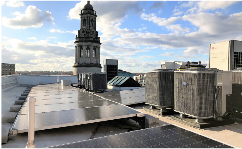
Rooftop solar panels cover the Pepco Resiliency Center at Maycroft Apartments, an affordable housing complex in Washington, D.C. Source: Timothy B. Wheeler, Bay Journal Media
