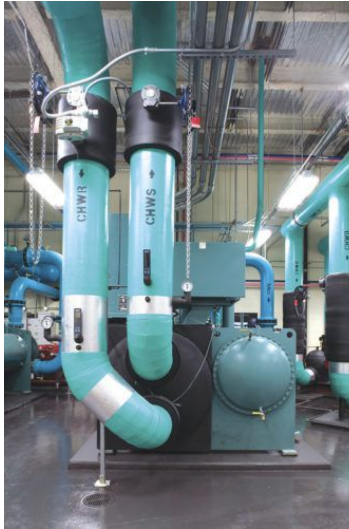
Figure 1: Any chiller that serves a hospital, which is a 24/7 critical load with a heavy energy demand, is a viable candidate for a chiller energy optimization system because chiller energy is a significant part of its operating costs. Courtesy: Smith Seckman Reid
