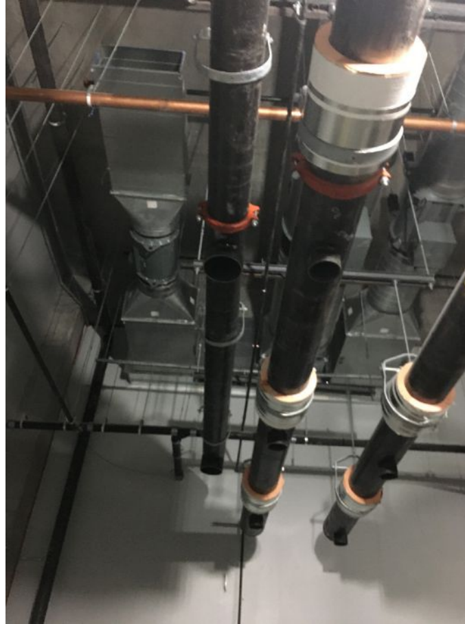
Figure 4: This is an example of a heating hot water header at primary system.
