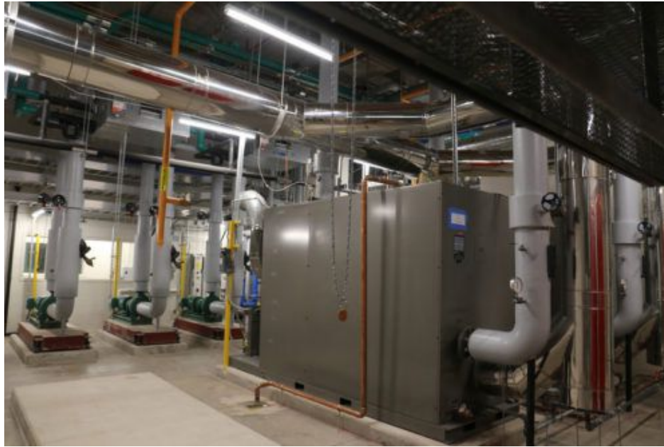
Figure 1: These are 6,000 MBH natural gas and oil dual fuel condensing boilers at the central plant for Texas Scottish Rite in Frisco, Texas. Courtesy: TDIndustries
