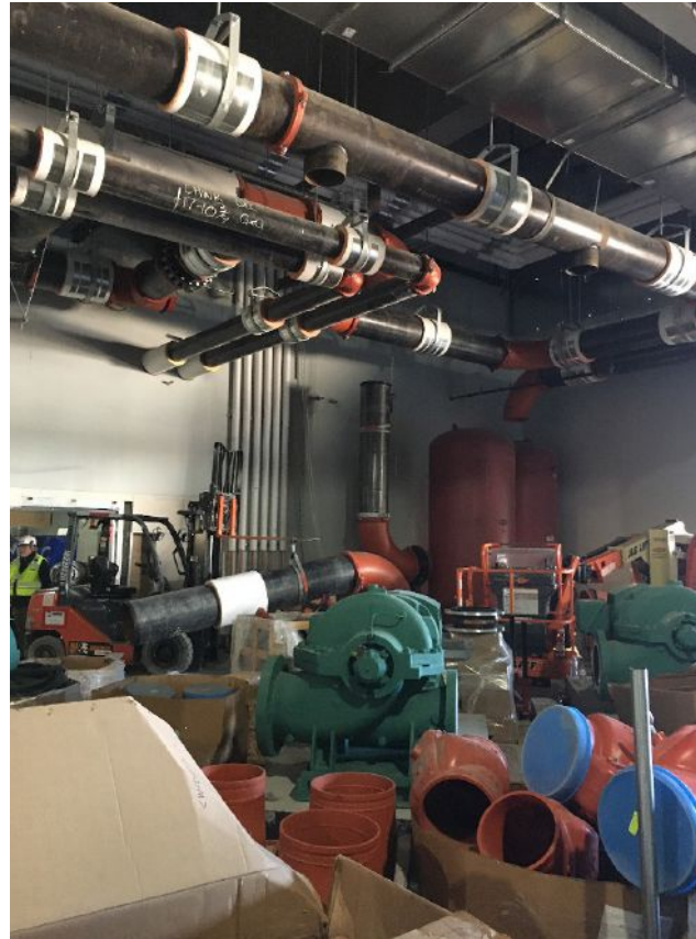
Figure 8: This shows a 20-inch chilled water pump header on secondary distribution system. Courtesy: ESD
