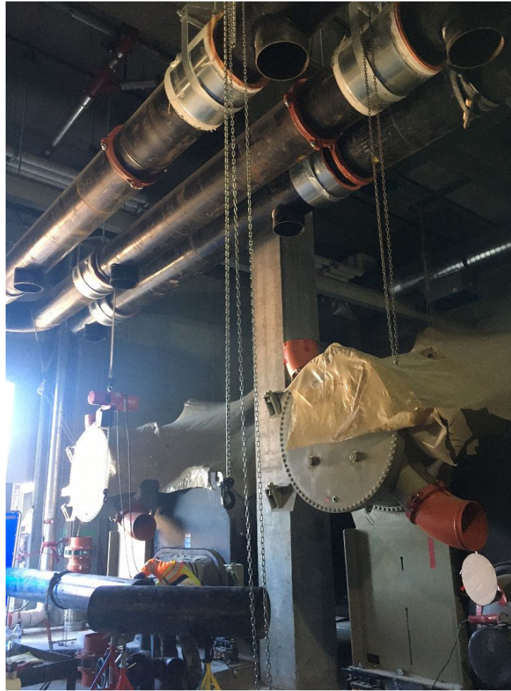
Figure 3: A 20-inch chilled water supply and return header is in a 7,000-ton central utility plant. Courtesy: ESD
