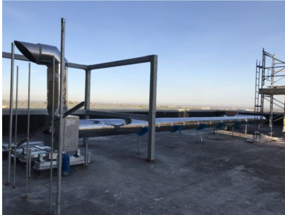
Figure 4: An exhaust fan serves a combined flue for dual fuel condensing boilers in a mechanical room. Courtesy: TDIndustries
