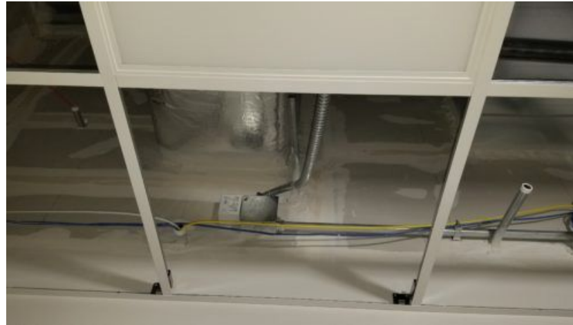
Figure 5: Image of a low-voltage lighting control relay with cabling installed in a haphazard method where the duct and ceiling tile will put strain on the connections. Courtesy: IMEG
