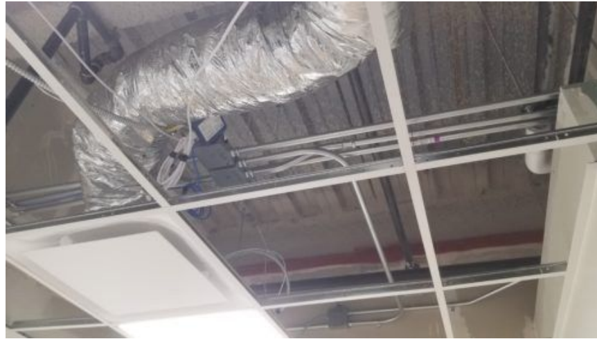
Figure 2: Image of a low-voltage lighting control relay connected to a junction box. Courtesy: IMEG
