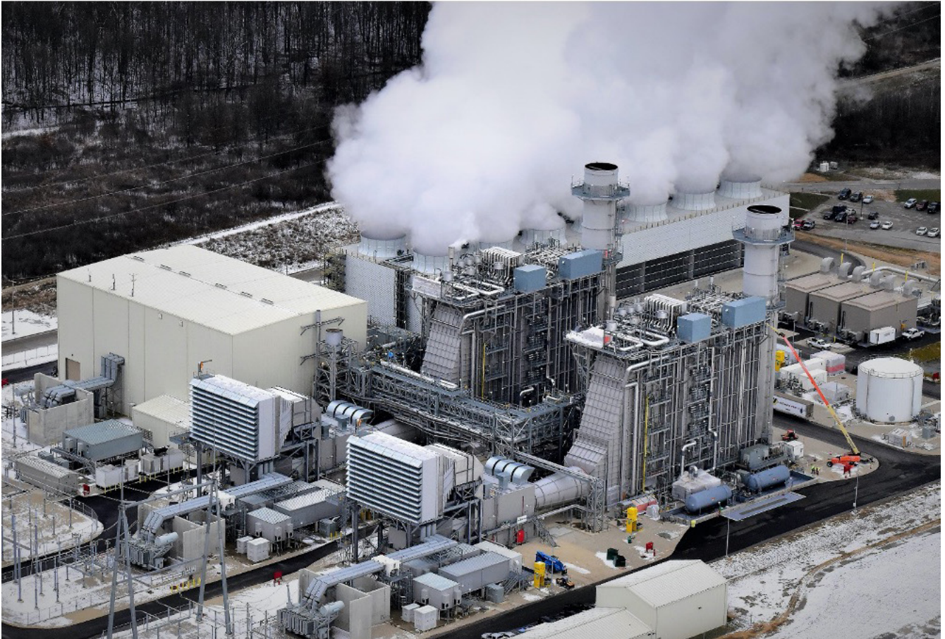
Figure F.2 Natural gas fueled combined cycle plant equipped for winter operation in the United States.
