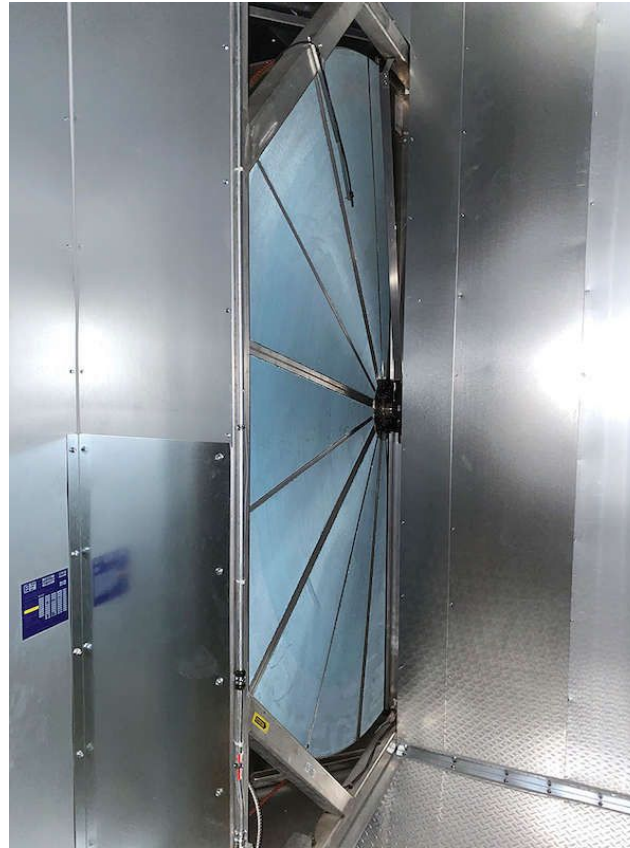
Figure 1: A total enthalpy wheel installed rooftop unit can provide additional energy savings. Courtesy: SmithGroup
