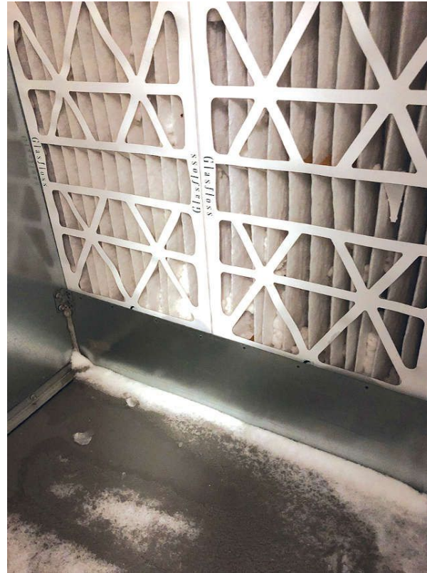
Figure 5: Designing the outdoor air plenum with a vertical chamber with an upward airflow velocity of less than 200 fpm will prevent snow from rising up and into the outdoor air ductwork. Courtesy: Peter Basso Associates
