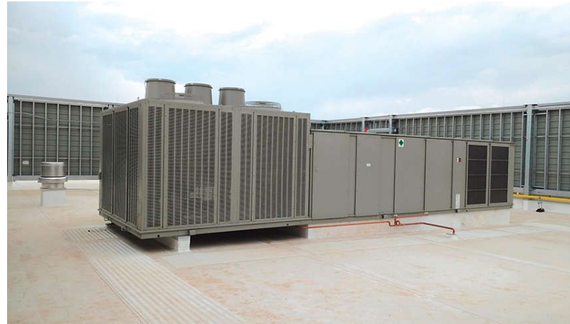
Figure 3: An air-cooled package rooftop unit shows lab exhaust stacks in the background. Courtesy: SmithGroup
