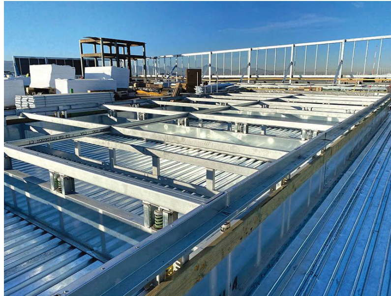
Figure 4: A vibration curb is used to isolate a rooftop unit from transmitting sound and vibrations to the building structure. Courtesy: SmithGroup
