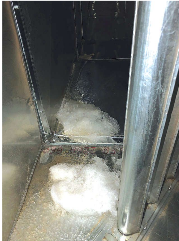
Figure 4: Snow entrained in the outdoor air flow can travel all the way into the air handling unit where it can plug filters and melt and cause damage to the AHU. Courtesy: Peter Basso Associates
