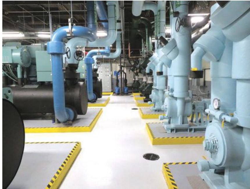
Figure 1: This photograph shows a 2,100-ton cooling plant serving a multitenant commercial office high-rise building. Courtesy: Raths, Raths & Johnson Inc.
