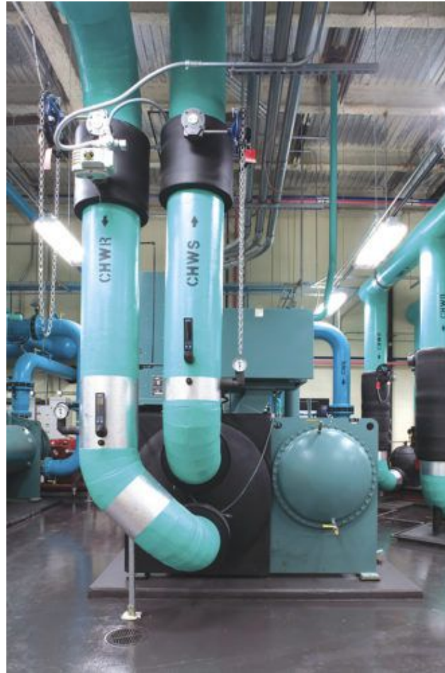
Figure 1: Any chiller that serves a hospital, which is a 24/7 critical load with a heavy energy demand, is a viable candidate for a chiller energy optimization system because chiller energy is a significant part of its operating costs. Courtesy: Smith Seckman Reid
