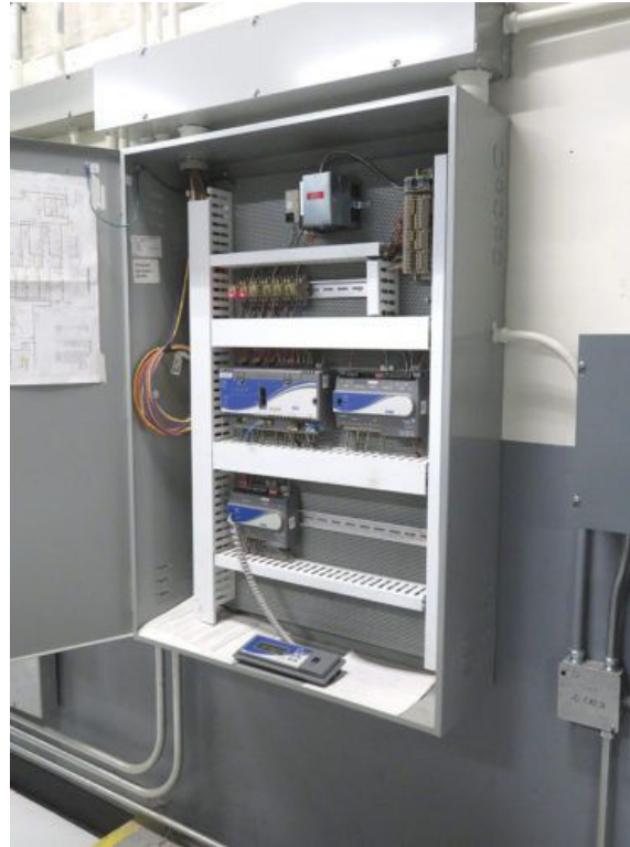
Figure 2: A cooling plant optimization controller is mounted in the plant adjacent to the chillers. Courtesy: Raths, Raths & Johnson Inc.
