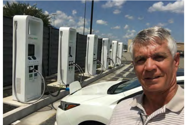
A Level 3 Charging Station in Breaux Bridge, Louisiana.
