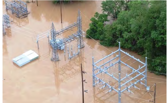
Flooded Clendenin Station in Kanawha County, West Virginia.
