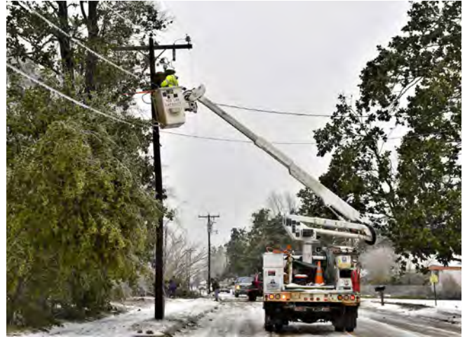
The severe winter weather in February 2021 that affected Texas and surrounding states serves as a cautionary tale of the effects extreme weather can have on energy facilities and supplies.
