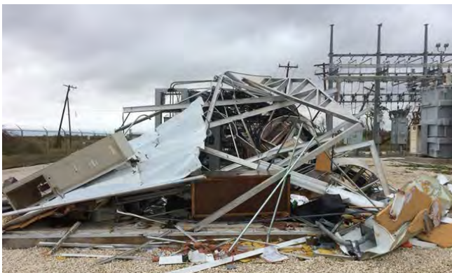
The photos show catastrophic wind damage to the Tatton Substation in Texas from Hurricane Harvey.
