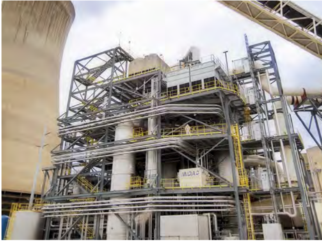
AEP's 20 MW CCUS project at the Mountaineer Plant in West Virginia validated the technology but was very expensive and disallowed by regulators in Virginia.
