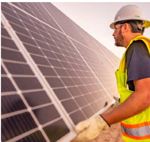
Image courtesy of Enel Green Power
