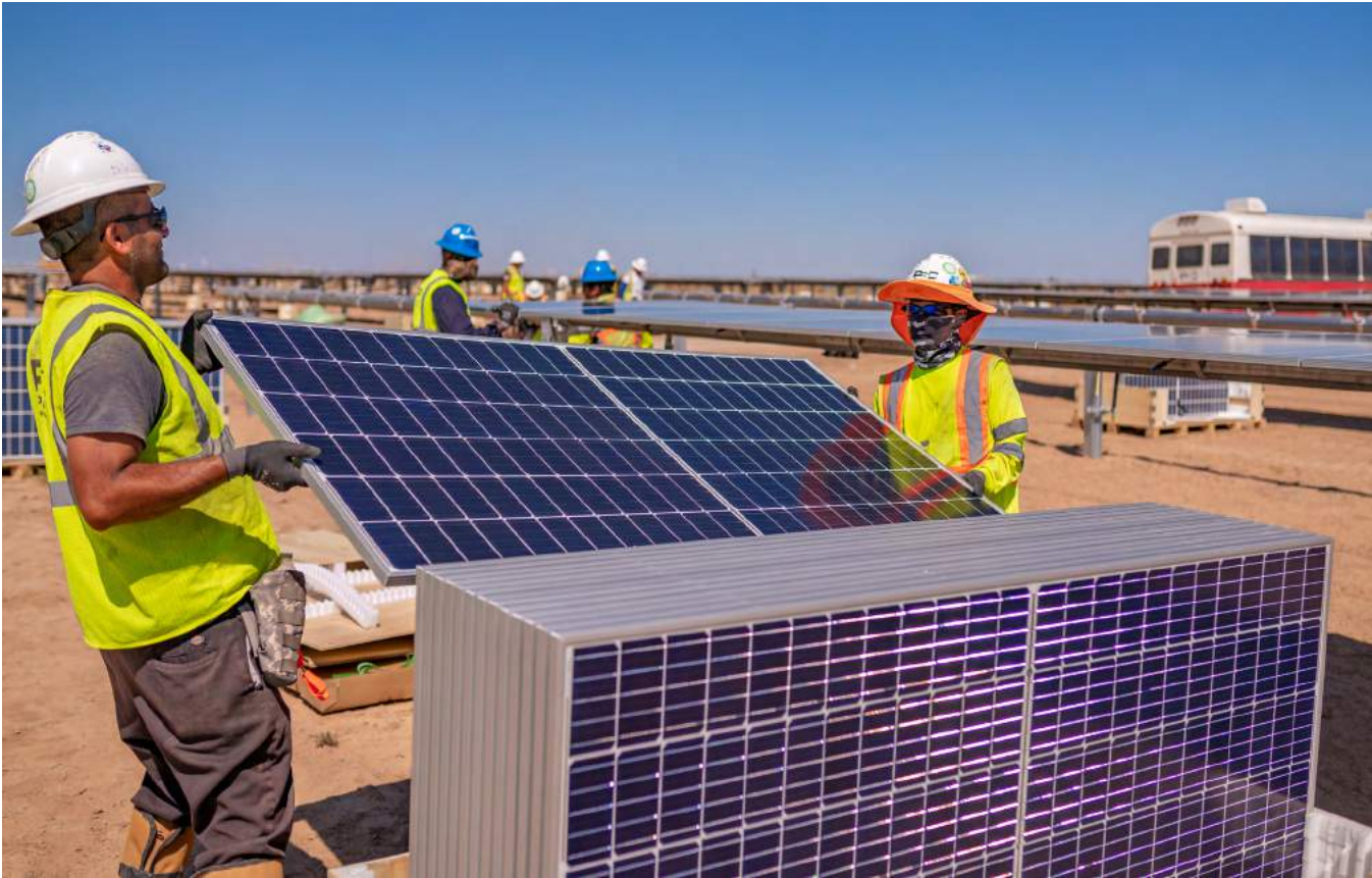
Image courtesy of Enel Green Power
