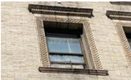
Existing Window: Most windows of this period have limited thermal breaks and poor airtightness, contributing to comfort problems year round. Photo Credit: Steven Winter Associates
