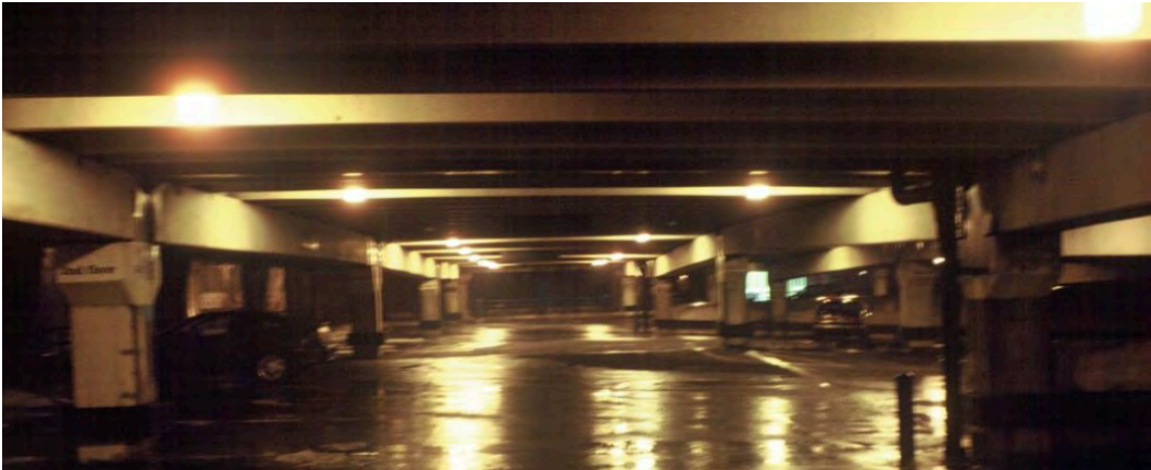
Bright, widely spaced luminaires in this parking garage create glare and deep shadows that can actually decrease safety. (NBI's Advanced Lighting Guidelines)
