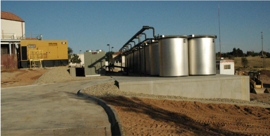
Figure 1. Thermal Storage System at the Amarillo, VA
