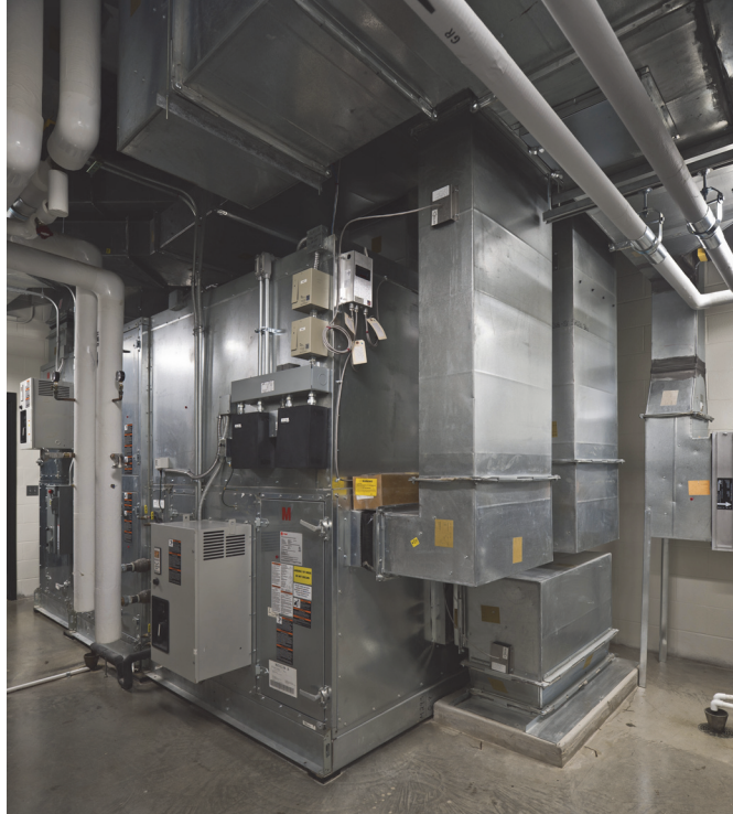
Figure 5-47 (HV15) DOAS unit with water coil. Photo reprinted with permission of CMTA
