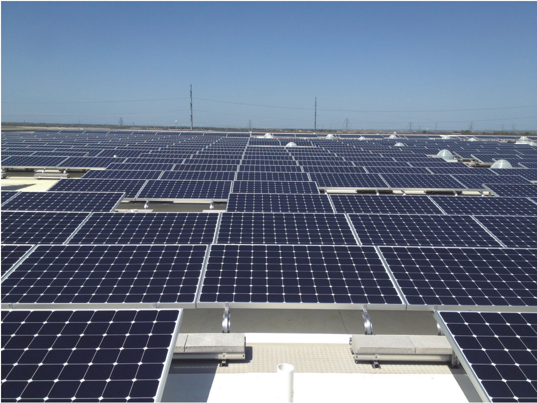
Figure 5-52 (RE5) Roof-mounted PV system. Photo reproduced by permission of Stantec
