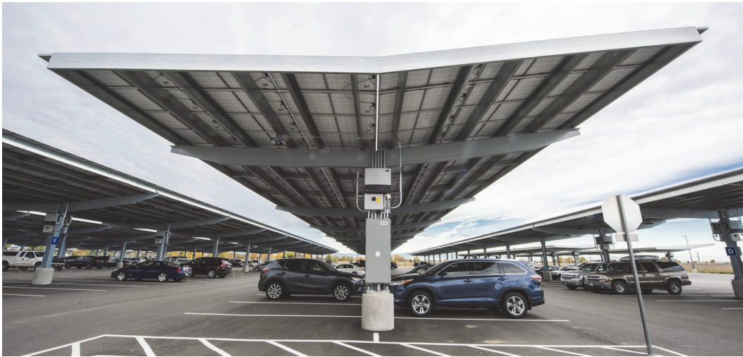
Figure 5-53 (RE5) PV canopy-mounted PV system. Photo by Dennis Schroeder, NREL Image 48750
