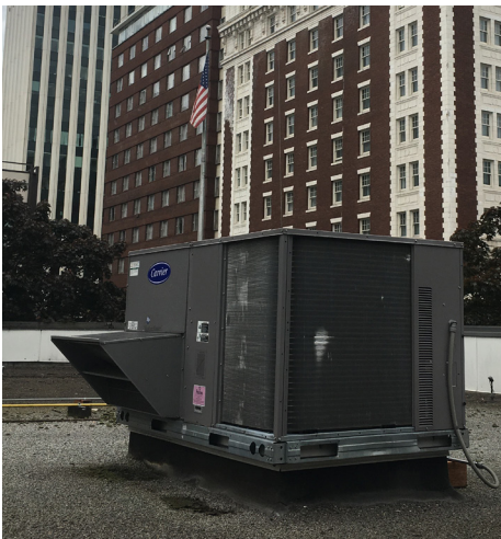
Rooftop air conditioner | Portland, OR Credit: Alexi Miller
